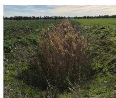
Figure 2: Unmaintained open ditch invaded by reeds: Tobias perimeter (Askri, 2021).
